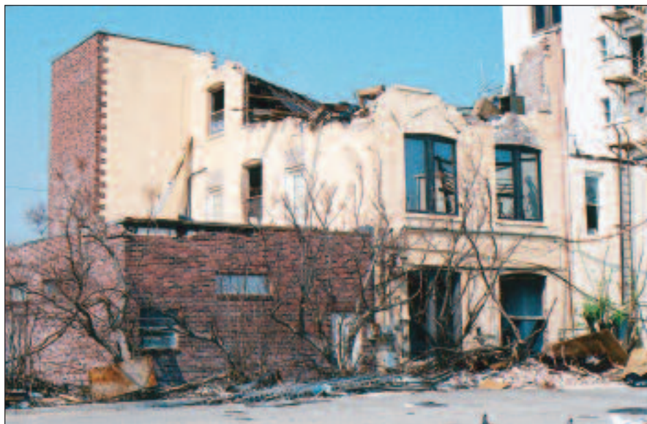
Damage caused by Hurricane Katrina to Gulfport attorney James Thompson's office building.
